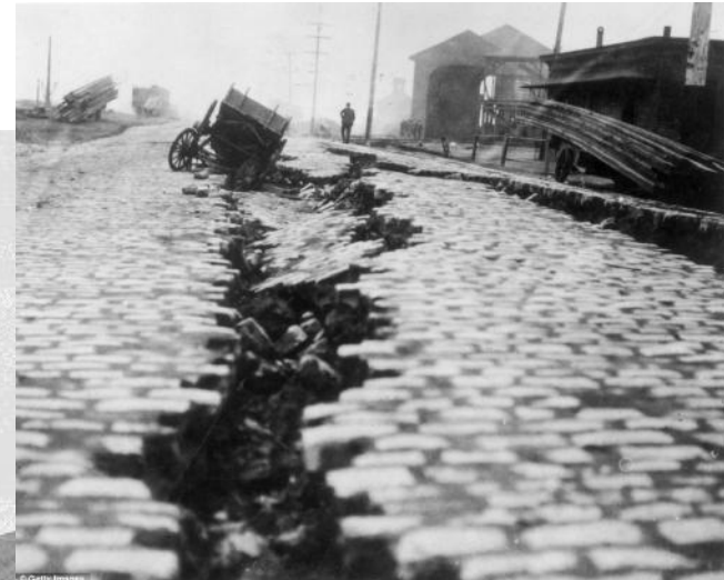
A cobblestone street, which was split down the middle after the Great Earthquake in San Francisco, California, in 1906
